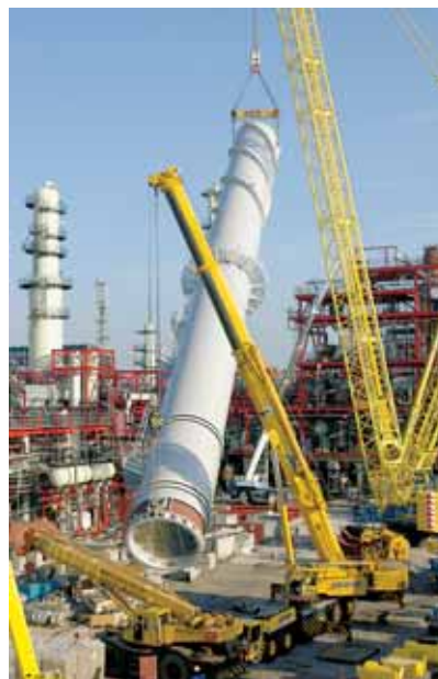
The new diesel production line will be completed at the Porvoo refinery by the end of 2006.
