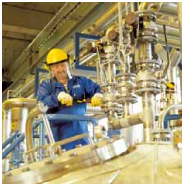
Kemira seeks growth in pulp and paper chemicals, water treatment chemicals, and paints and coatings. The company has production sites in over 30 countries. The picture shows Kemira's plant in Oulu, where the main products are hydrogen peroxide and formic acid.
